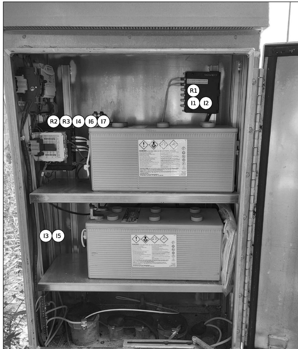
TYPICAL EXISTING SOLAR CABINET
