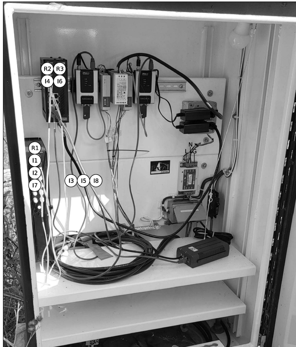
TYPICAL EXISTING CCTV/RTMS CABINET
