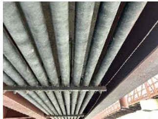
EXISTING AT&T STEEL CONDUITS MOUNTED TO UNDERSIDE OF DEERFIELD ROAD BRIDGE OVER DES PLAINES RIVER
