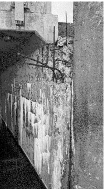
Picture of damage at North corner of West Abutment
