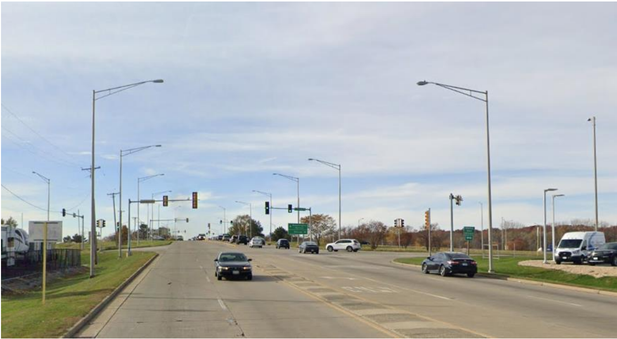
Existing IDOT interchange lighting along US 52 at East Frontage Road (looking west).
