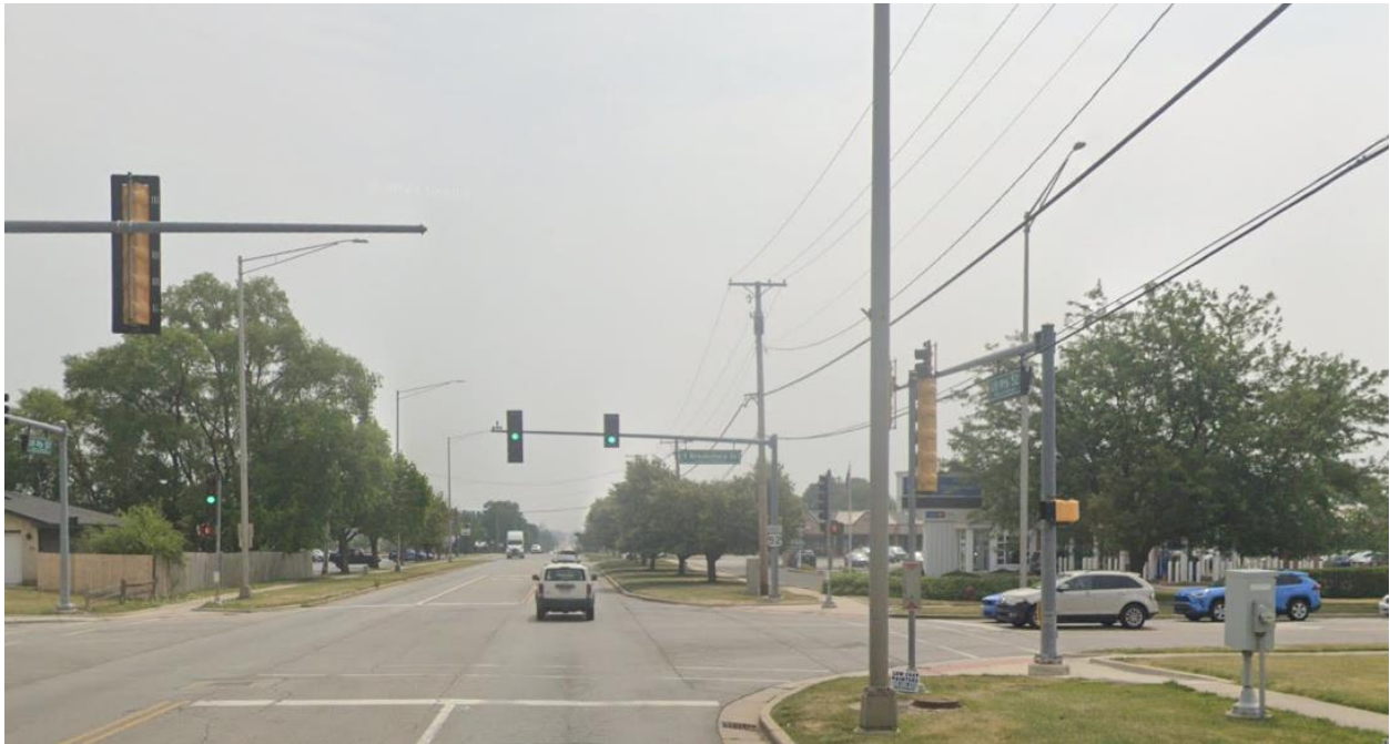
Signalized intersection of US 52 and Brookshore Drive (looking East) showing Village of Shorewood Brookshore lighting system. Note pedestal mounted lighting controller on the intersection's southwest corner.
