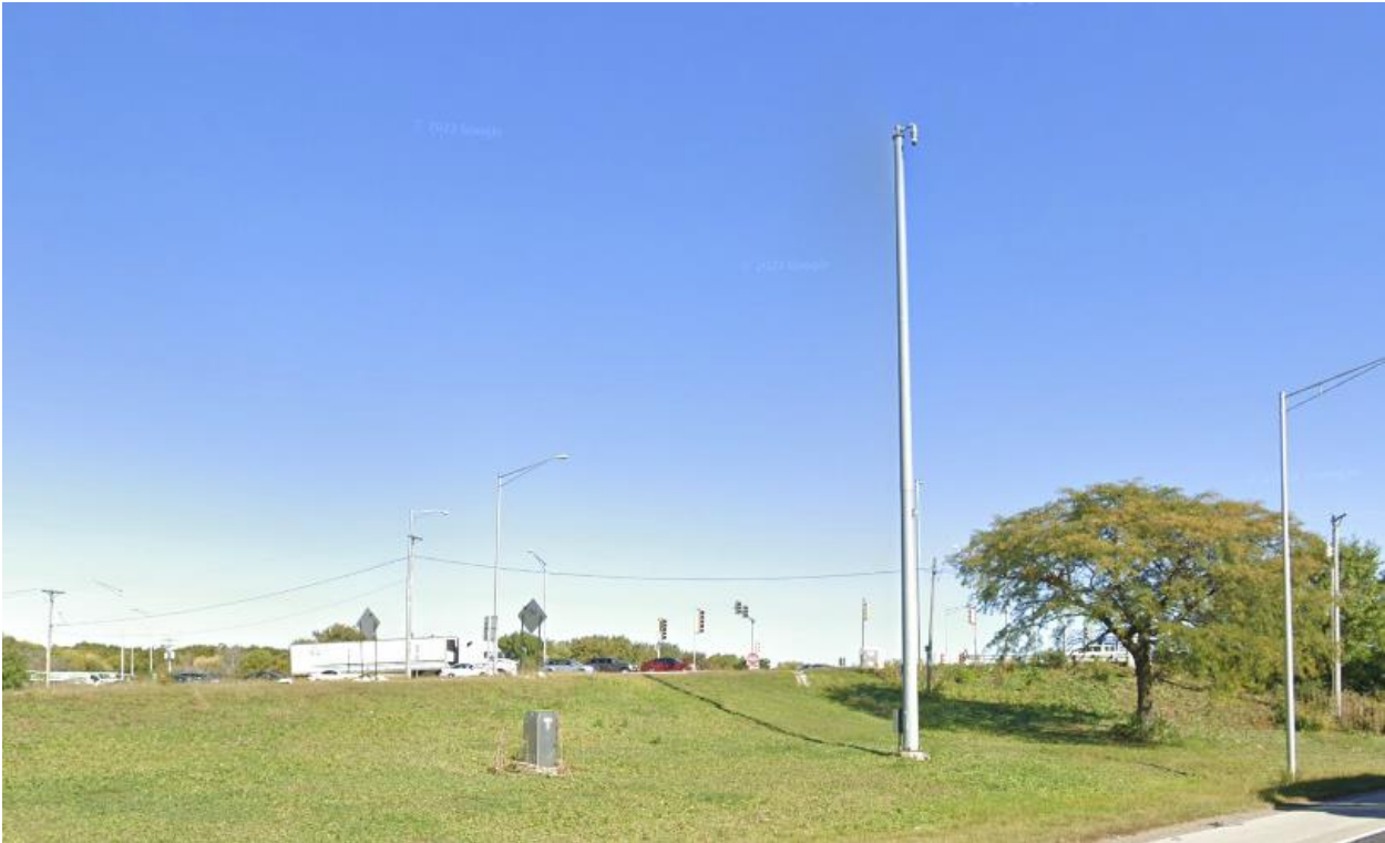
Existing IDOT CCTV Camera on 80-ft pole and ITS cabinet (southwest infield interchange quadrant).
