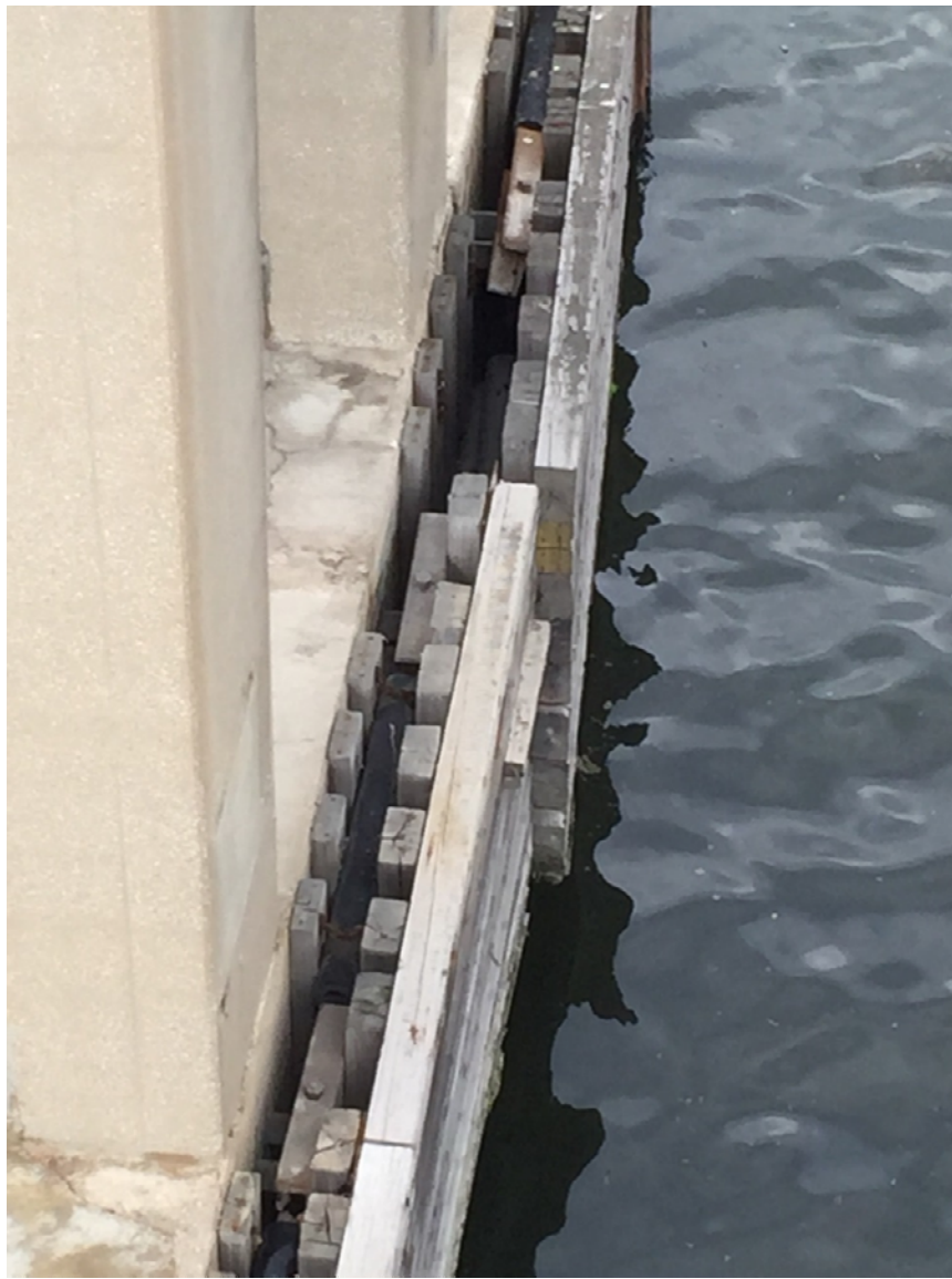
SN 016-0487 – Pier 15 – Detached Fender System Panel
