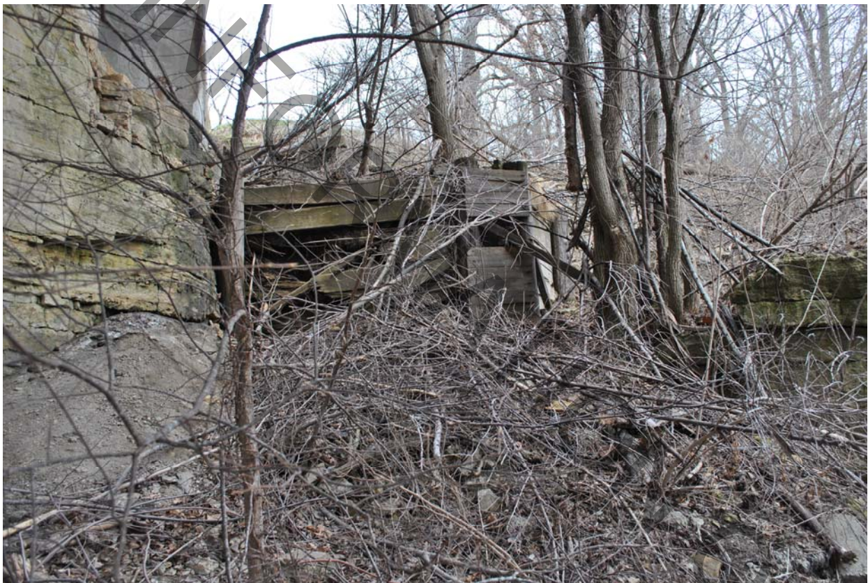
Figure 4: Picture of wooden retaining structure in the NW quadrant of the west abutment.
