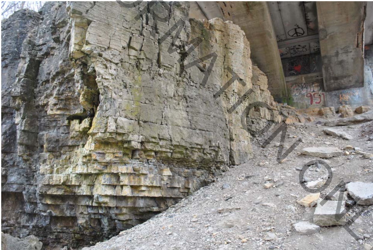
Figure 3: Picture of the rock formation in front of the east abutment of SN046-0065.
