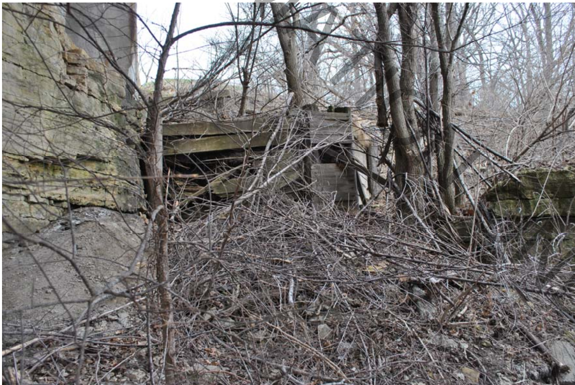
Figure 9: Failing wood retaining wall immediately north of west abutment.
