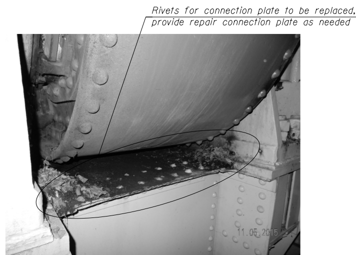
PHOTO 1: NORTH TRUSS CONNECTION PLATE (NW corner shown, SW corner and NE corner similar)
