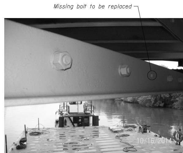
PHOTO 13: BOTTOM DIAGONAL LATERAL BRACING ANGLE CONNECTION (Between Floorbeams 7 and 8 - WEST LEAF)
