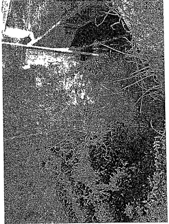
SCOUR HOLE AT DOWNSTREAM END STRUCTURE NO. 083-2019 OVER CREEK
