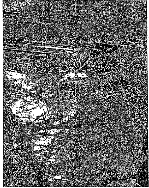
LOOKING DOWNSTREAM IN FRONT OF WEST PIER STRUCTURE NO. 044-0027 OVER BAY CREEK
