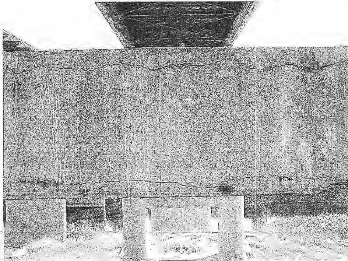
Pier 1A cracking SECOND FROM TOP DIAPHRAGM
