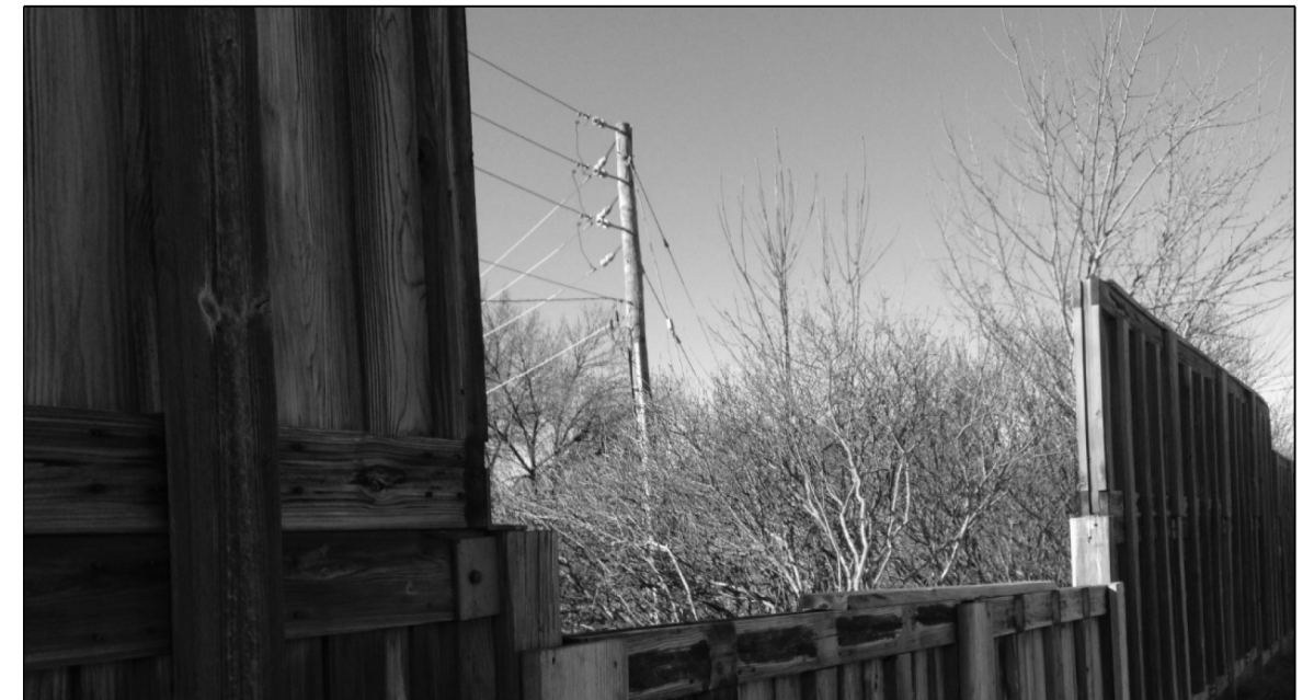
LOC. 1A: WOOD NOISE WALL REPLACE 17 FT WIDE X 9 FT TALL OF NOISE WALL
