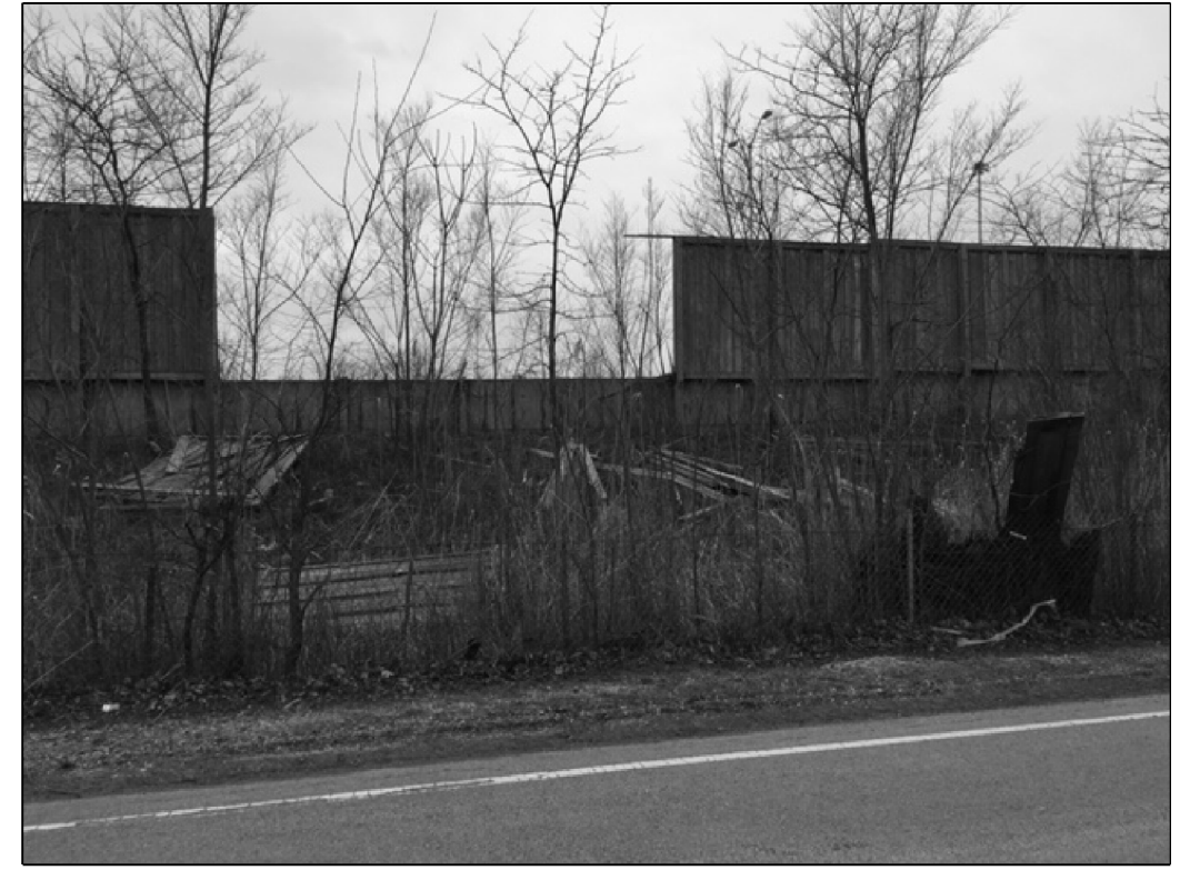
LOC. 7A : WOOD NOISE WALL MOUNTED TO THE CONCRETE BARRIER WALL REPLACE 33.5 FT WIDE X 15 FT TALL OF NOISE WALL SEE SHEET 17A FOR PANEL INFORMATION.
