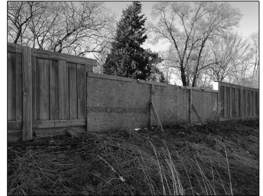
LOC. 1 : WOOD NOISE WALL REPLACE 24 FT WIDE X 5 FT TALL OF NOISE WALL
