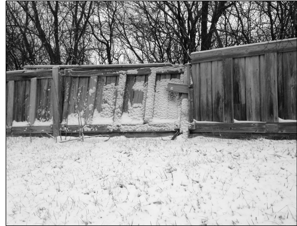
LOC. 1B: WOOD NOISE WALL REINSTALL 17 FT WIDE X 4'-7" TALL OF NOISE WALL
