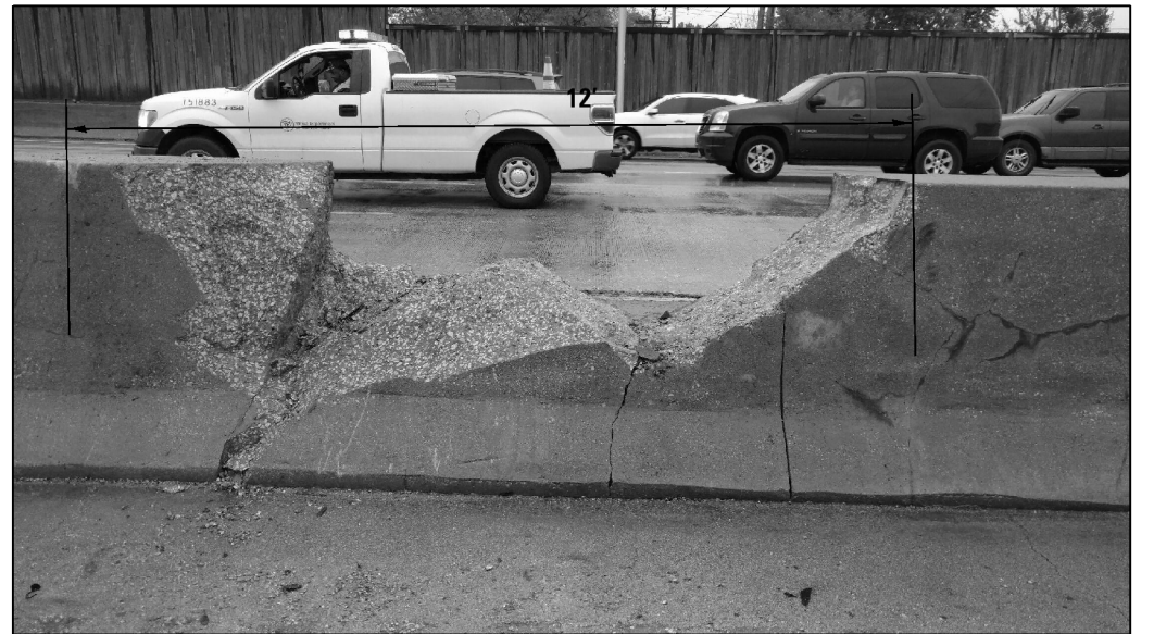
FULL DEPTH REPAIR (LOC.7) REPLACE 12 FT OF BARRIER WALL FOR MORE DETAILS SEE SHEET #6
