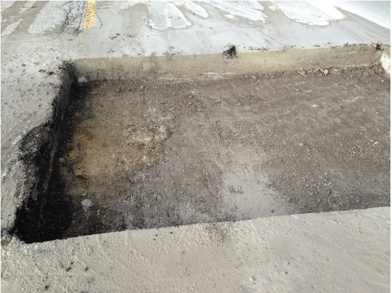
Photo 1: Example of a typical patch with a subbase in good condition.
