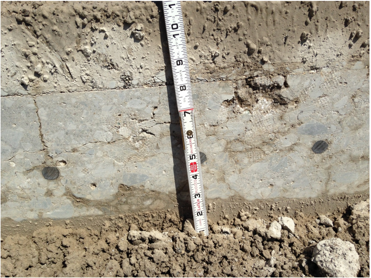
Photo 3: Example of typical D cracking of the PCC pavement in Section 53-4.
