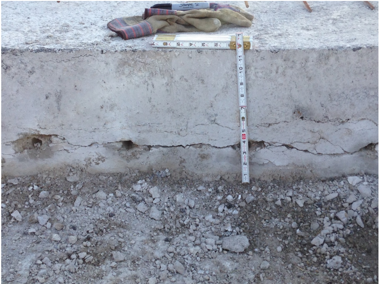
Photo 4: Example of typical D cracking with a horizontal crack in the PCC in Section 53-4.
