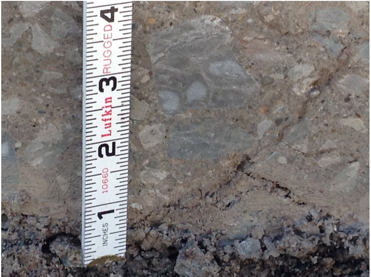
Photo 2: Example of typical cracking in the aggregate in Section 53-4.
