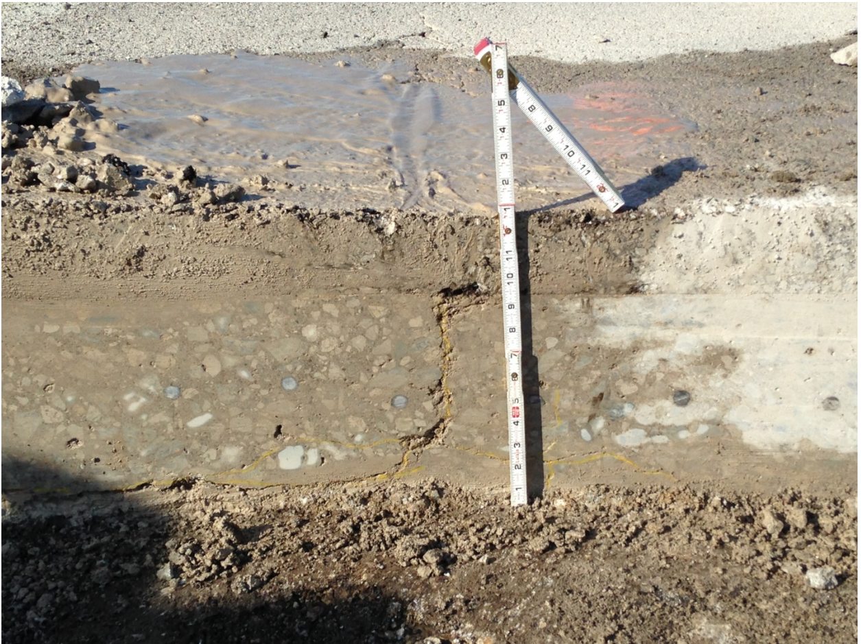
Photo 5: Example of a reflective longitudinal crack in the HMA overlay caused by an underlying longitudinal crack in the PCC pavement in Section 53-4.
