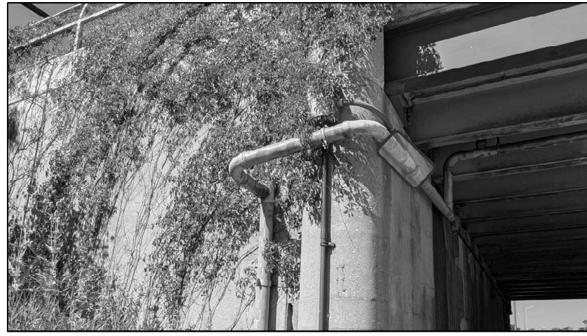
016-2036 PHOTO #1 SOUTH ABUTMENT EAST CORNER REPLACE LONGITUDINAL SECTION, 4 FEET
