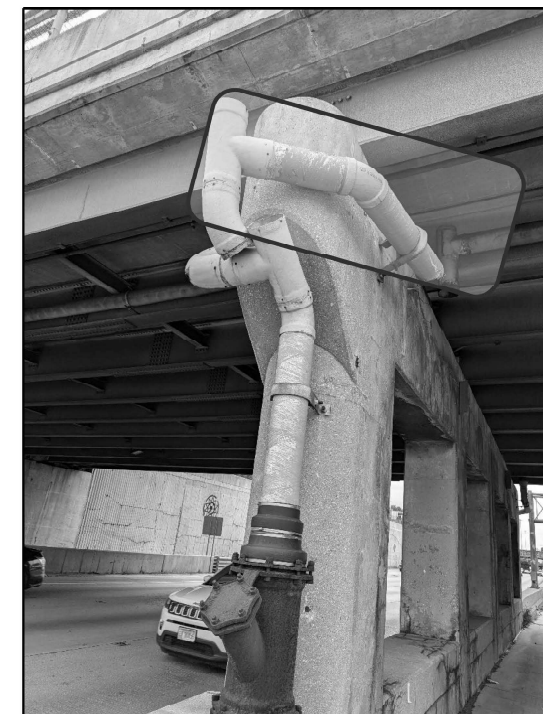
016-1151 PHOTO #2 PIER 4 NORTH END REPLACE FROM LONGITUDINAL RUN TO DOWNSPOUT, 12 FEET
