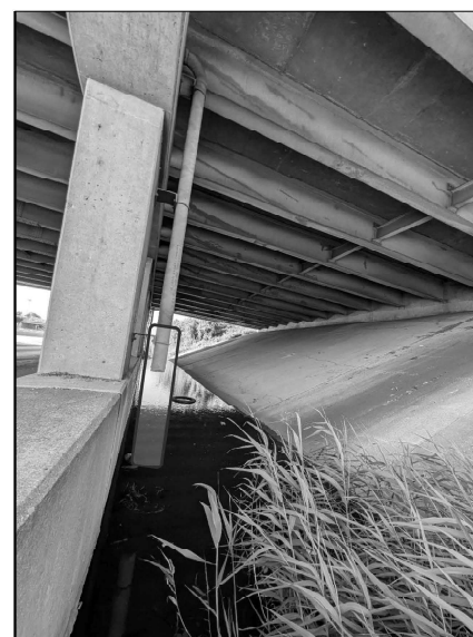
016-1145 PHOTO #1 NORTHWEST CORNER OF BRIDGE REPLACE BOTTOM OF DOWNSPOUT AT NORTHWEST CORNER, 4 FEET
