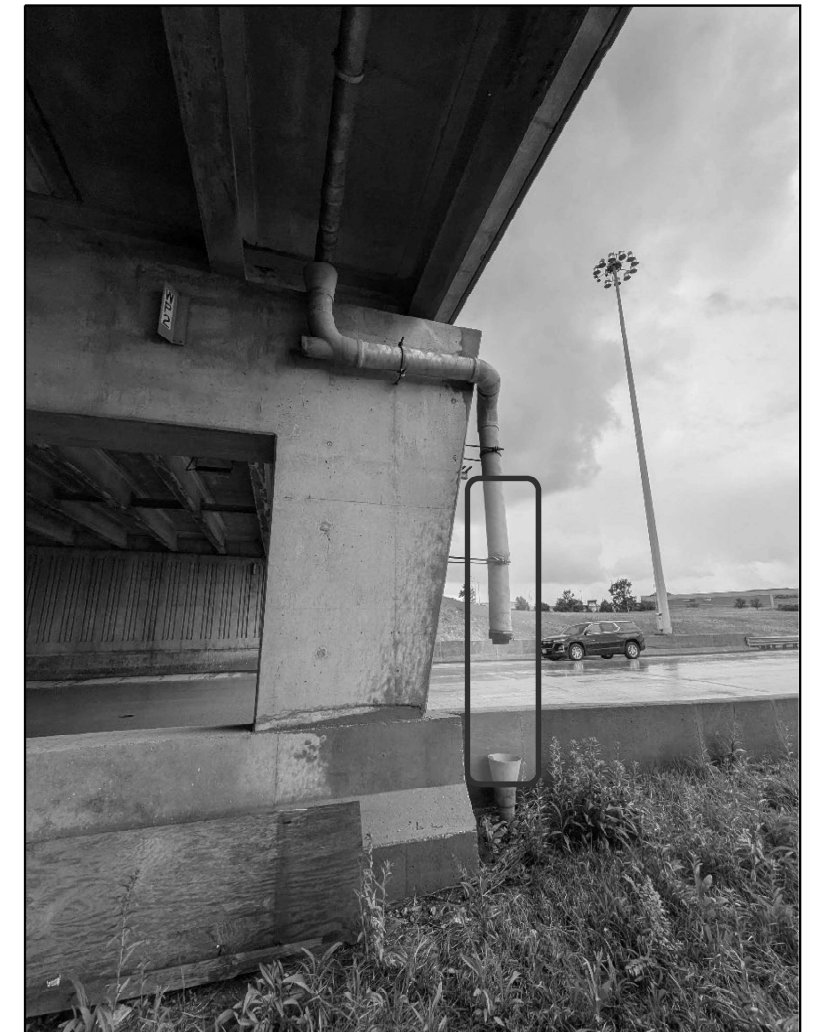
016-2760 PHOTO #1 PIER 1 WEST END REPLACE DRAIN PIPE CONNECTION TO INLET, 8 FEET
