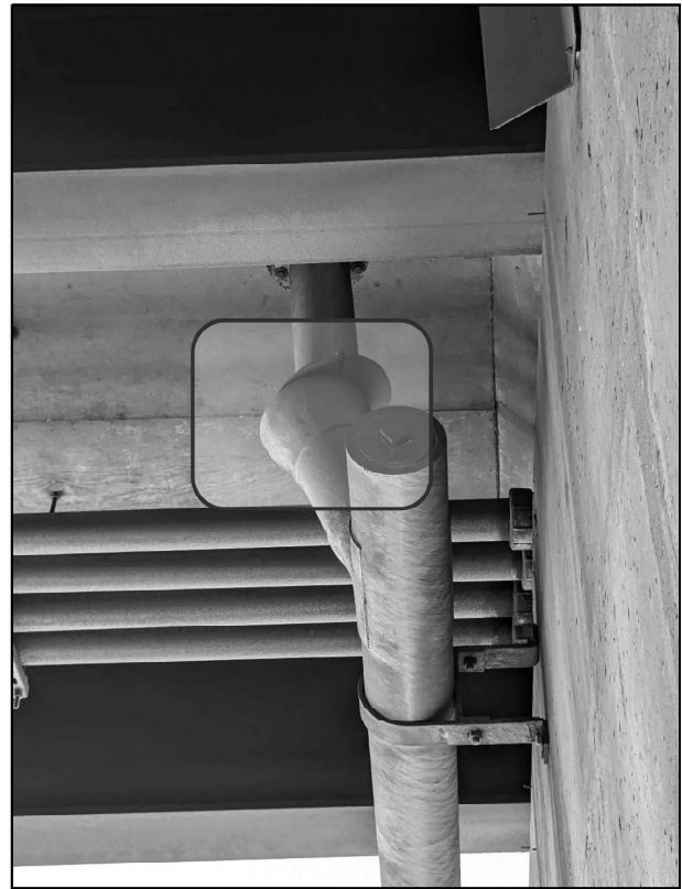
016-1143 PHOTO #2 SOUTHWEST CORNER OF BRIDGE REALIGN DOWNSPOUT TO DRAINPIPE CONNECTION, 2 FEET
