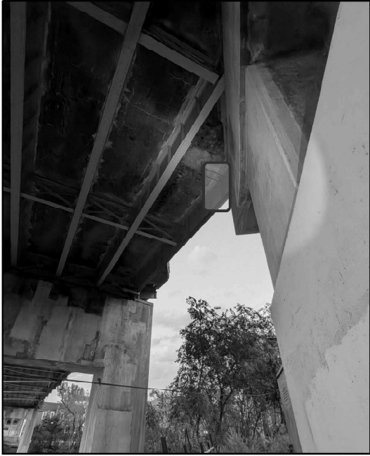
016-0777 PHOTO #3 SPAN 10 WEST SIDE - NEAR PIER 11 - DRAIN PIPE 3 EXTEND PIPE TO 6 INCH BELOW BOTTOM FLANGE, 4 FEET
