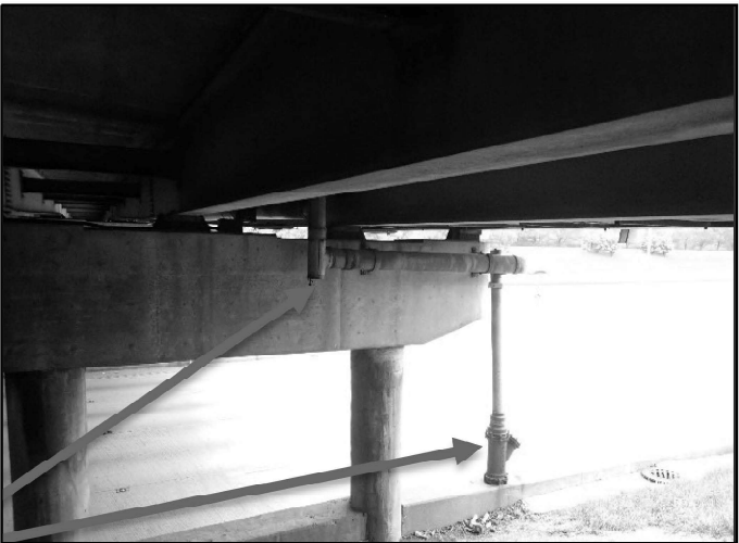
016-1160 PHOTO #6 PIER 1 SOUTH END DRAINAGE (FURTHEST WEST) MISSING PLUG AT BOTTOM & BROKEN CLAMP, 2 FEET
