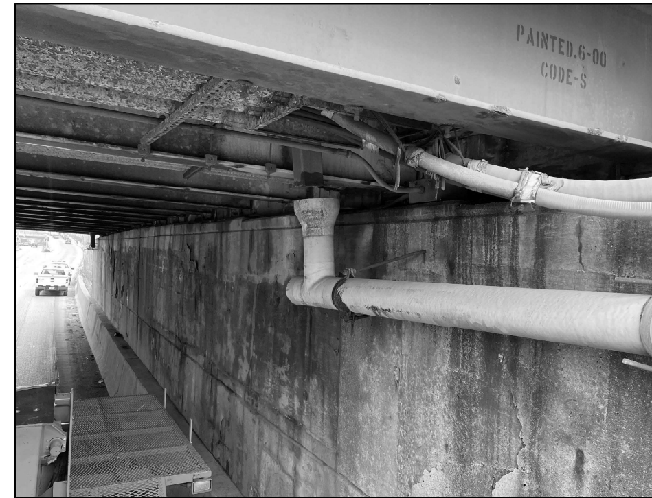
016-0189 PHOTO #3 EAST ABUTMENT DRAINAGE REPLACE PIPE SUPPORT CONNECTION AND RAISE THE FLARED END PIPE WHERE EXTENSION EXTENDS INTO FLARED PIPE TO ALLOW PROPER DRAINAGE, 2 FEET
