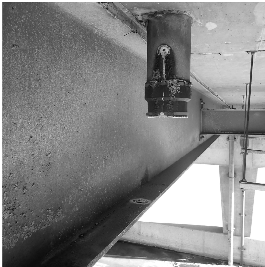
016-1145 PHOTO #2 SOUTHWEST CORNER OF BRIDGE EXTEND DRAINAGE PIPE TO 6 INCH BELOW BOTTOM FLANGE - 2 FEET
