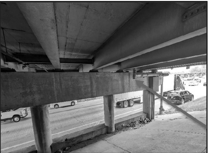
016-1160 PHOTO #4 PIER 5 NORTH END DRAINAGE (FURTHEST EAST) MISSING PLUG AT BOTTOM, 1 FEET
