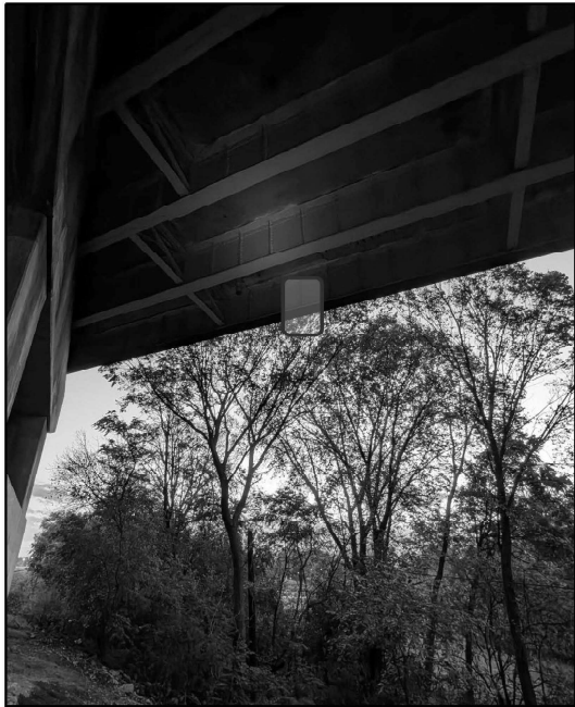
016-0777 PHOTO #5 SPAN 10 EAST SIDE - NEAR PIER 12 - DRAIN PIPE 5 EXTEND PIPE TO 6 INCH BELOW BOTTOM FLANGE, 4 FEET
