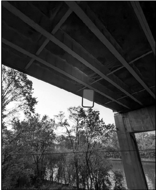
016-0777 PHOTO #4 SPAN 10 EAST SIDE - NEAR PIER 10 - DRAIN PIPE 4 EXTEND PIPE TO 6 INCH BELOW BOTTOM FLANGE, 4 FEET
