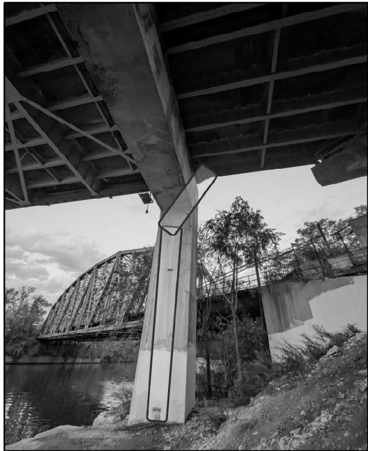
016-0777 PHOTO #1 PIER 10 WEST END - DRAIN PIPE 1 REPLACE EXTENSION TO THE GROUND, 40 FEET
