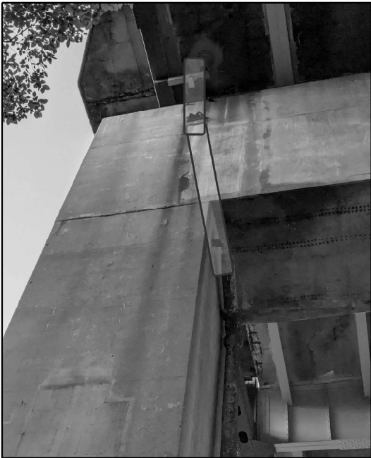
016-0777 PHOTO #2 PIER 10 EAST END - DRAIN PIPE 2 REPLACE EXTENSION TO GROUND, 15 FEET
