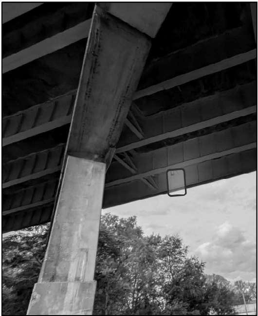
016-0777 PHOTO #7 SPAN 13 WEST SIDE - NEAR PIER 13 - DRAIN PIPE 7 EXTEND PIPE TO 6 INCH BELOW BOTTOM FLANGE, 4 FEET
