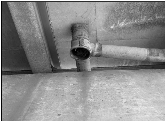
016-1160 PHOTO #5 PIER 5 NORTH END DRAINAGE (FURTHEST EAST) MISSING PLUG AT BOTTOM
