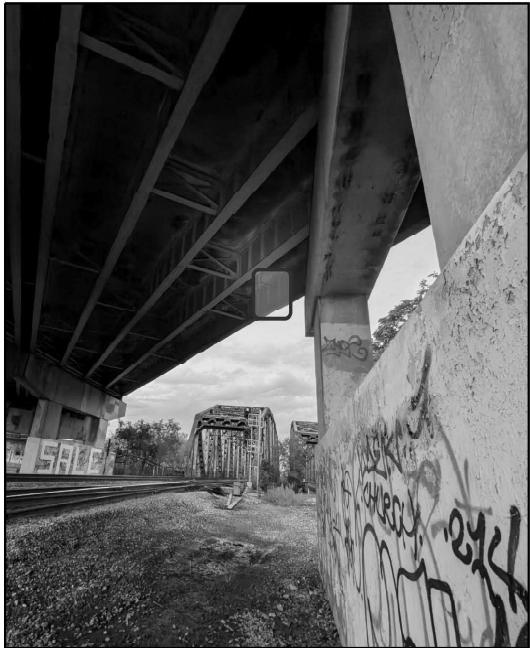
016-0777 PHOTO #6 SPAN 12 WEST SIDE - NEAR PIER 12 - DRAIN PIPE 6 EXTEND PIPE TO 6 INCH BELOW BOTTOM FLANGE, 4 FEET
