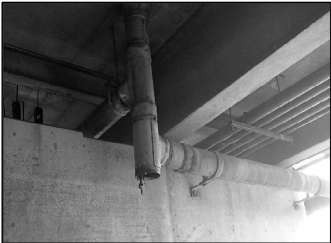
016-1160 PHOTO #7 PIER 1 SOUTH END DRAINAGE (FURTHEST WEST) MISSING PLUG AT BOTTOM
