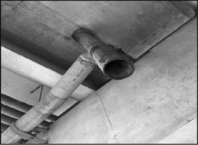
016-1160 PHOTO #3 PIER 5 SOUTH EAST DRAINAGE (FURTHEST EAST) MISSING PLUG AT BOTTOM
