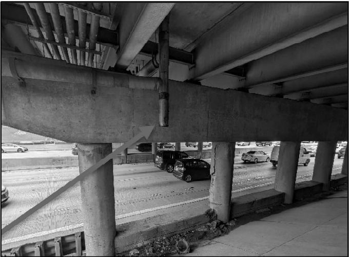
016-1160 PHOTO #2 PIER 5 SOUTH EAST DRAINAGE (FURTHEST EAST) MISSING PLUG AT BOTTOM, 1 FEET
