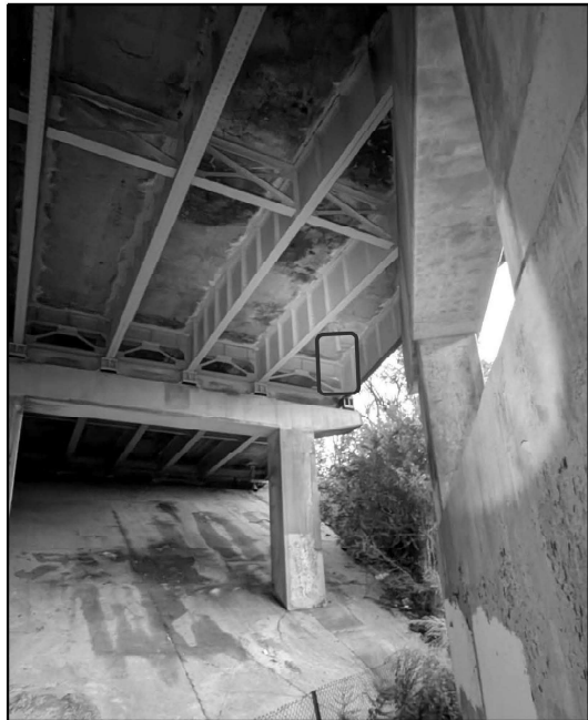
016-0777 PHOTO #9 SPAN 13 EAST SIDE - NEAR PIER 14 - DRAIN PIPE 9 EXTEND PIPE TO 6 INCH BELOW BOTTOM FLANGE, 4 FEET
