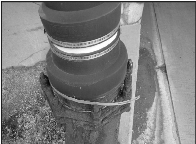
016-1160 PHOTO #8 PIER 1 SOUTH END DRAINAGE (FURTHEST WEST) BROKEN CLAMP
