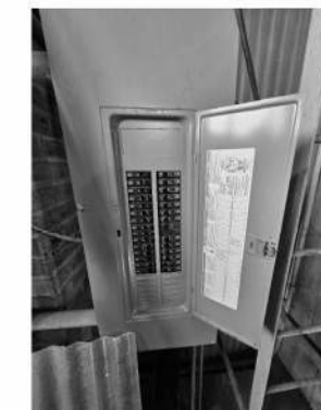
WEST BRIDGE HOUSE LIGHTING PANEL 120/280V, 3-PHASE, 4-WIRE
