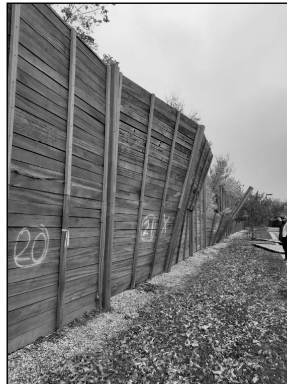
TYPICAL WALL POST AND PANEL DAMAGE (Looking from residential side)
