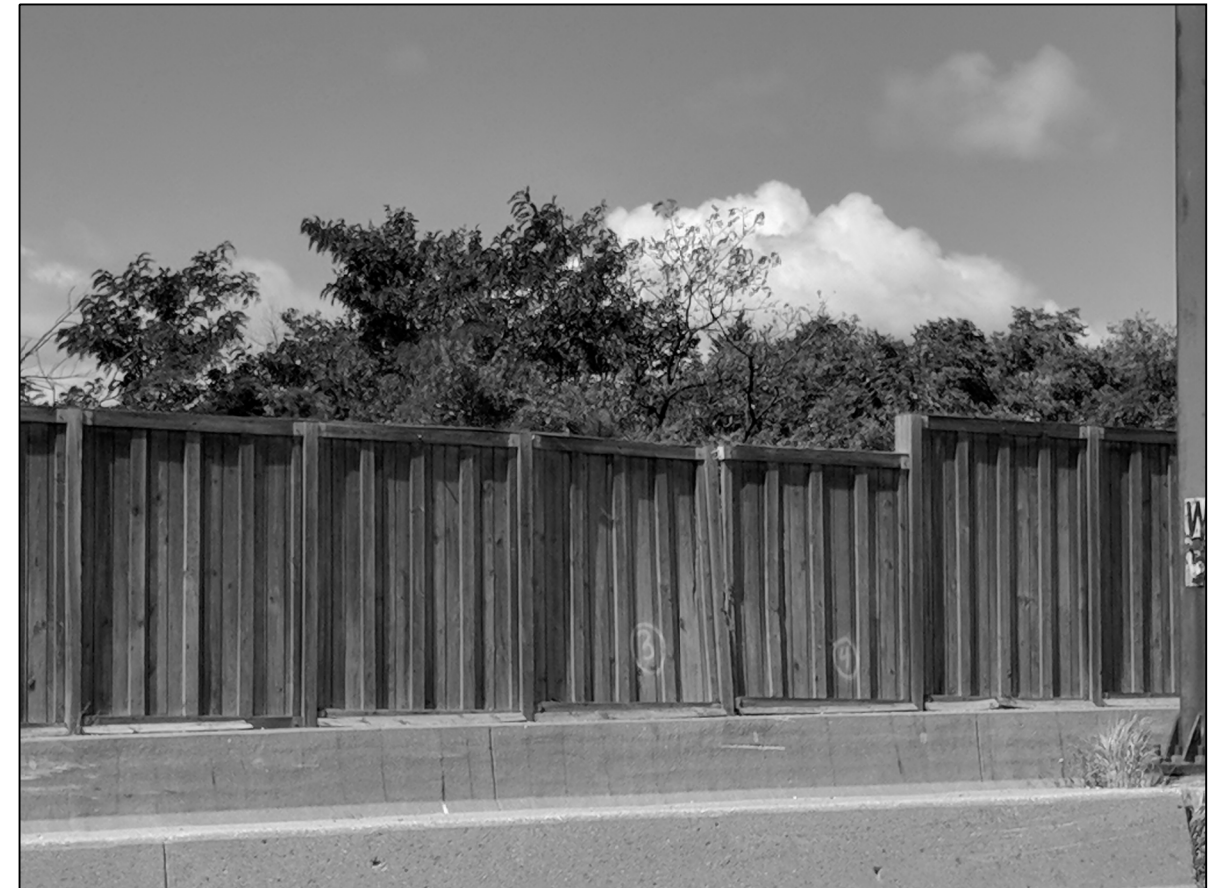
LOC. 26: DOUBLE SIDED WOODEN SOUND WALL PANELS. REPLACE 7.5 FT X 9 FT-7 IN (H) OF WOODEN WALL PANELS ON TOP OF CONCRETE BARRIER WALL (2 PANELS # 3 & 4)
