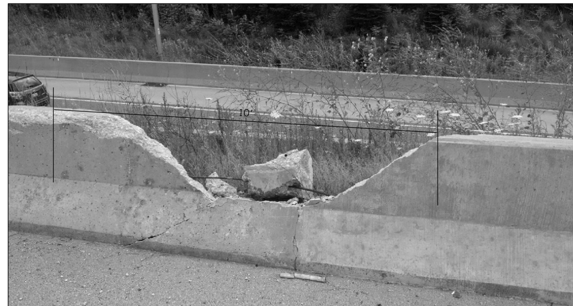
FULL DEPTH REPAIR REPLACE 10 FT OF BARRIER WALL LOC.12 FOR MORE DETAILS SEE SHEET #6
