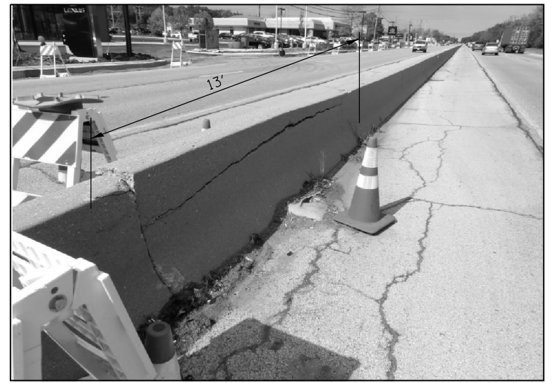
FULL DEPTH REPAIR REPLACE 13 FT OF BARRIER WALL LOC. 8 FOR MORE DETAILS SEE SHEET #6
