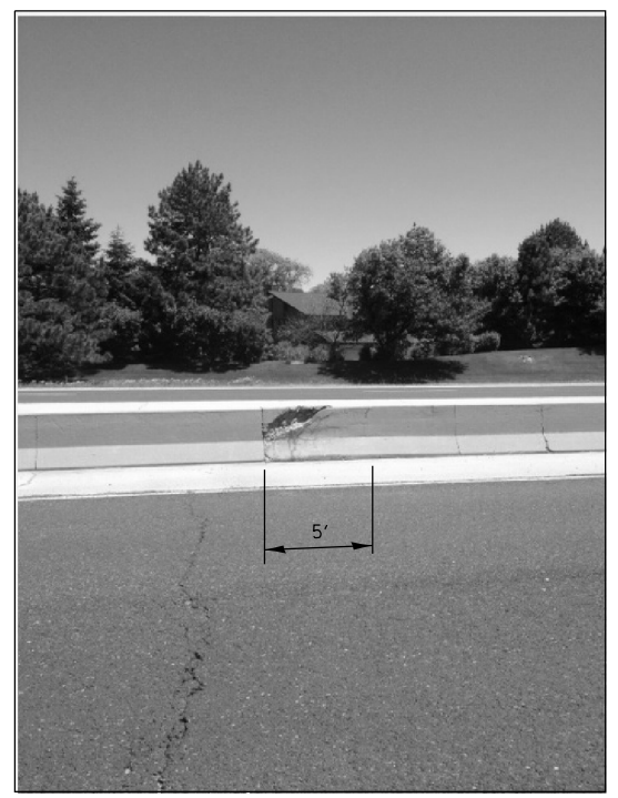
FULL DEPTH REPAIR REPLACE 5 FT OF BARRIER WALL LOC. 6 FOR MORE DETAILS SEE SHEET #6
