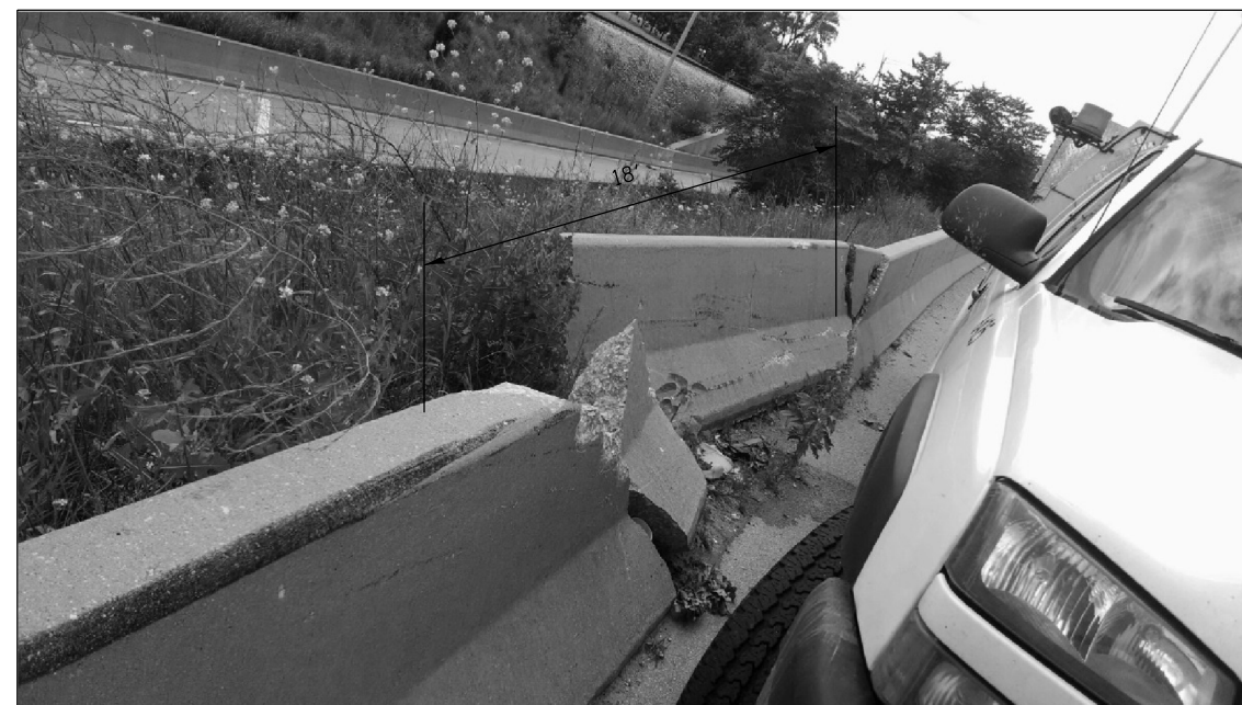
FULL DEPTH REPAIR REPLACE 18 FT OF BARRIER WALL LOC. 13 FOR MORE DETAILS SEE SHEET #6
