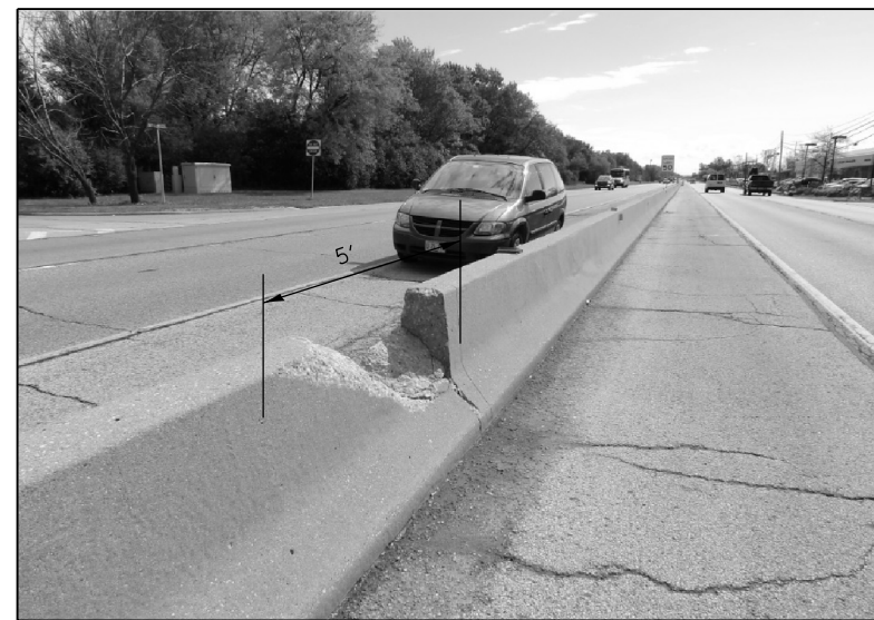
FULL DEPTH REPAIR REPLACE 5 FT OF BARRIER WALL LOC. 9 FOR MORE DETAILS SEE SHEET #6
