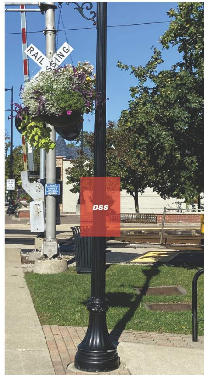
New sign panel mounted on existing light pole below height restriction sign.
