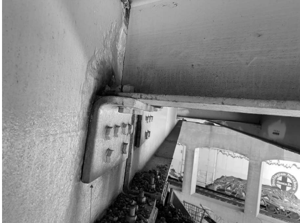
R2 Picture 4: P2; Beam 6 West Face
