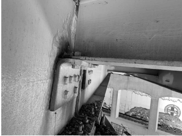
R2 Picture 4: P2; Beam 6 West Face
