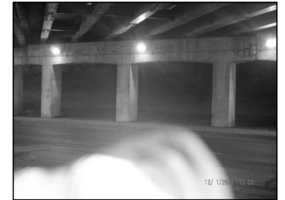
EXISTING LIGHTING: PIER 1 (Looking Southeast)
