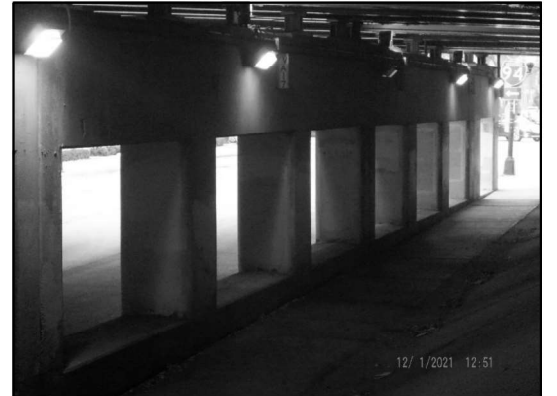
EXISTING LIGHTING: PIER 1 (Looking Southwest)
