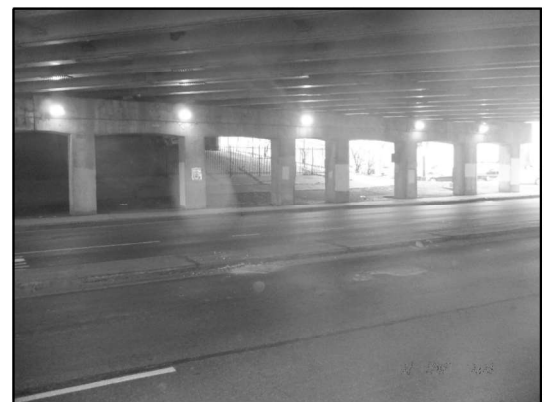
EXISTING LIGHTING: PIER 1 (Looking Southwest)
