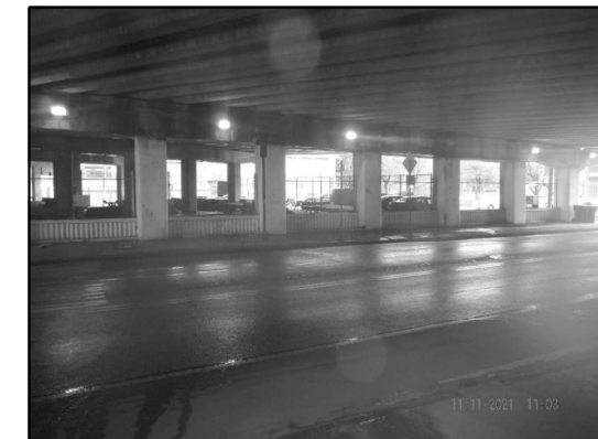
EXISTING LIGHTING: PIER 23 (Looking Southwest)
