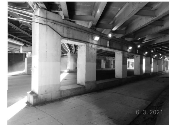
EXISTING LIGHTING: Pier 2 (Looking East)
