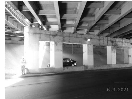
EXISTING LIGHTING: PIER 1 (Looking West)
