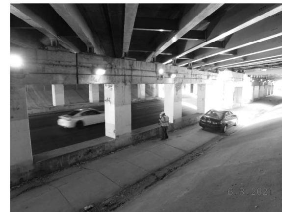
EXISTING LIGHTING: PIER 1 (Looking East)
