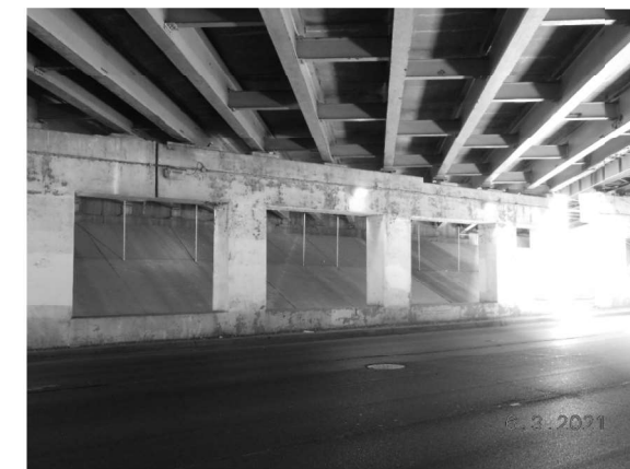
EXISTING LIGHTING: Pier 2 (Looking West)
