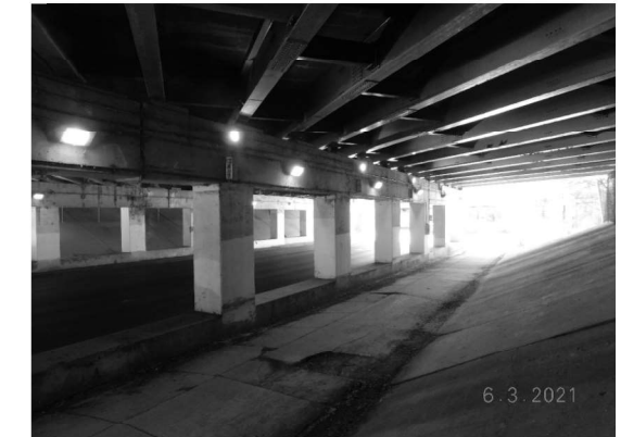
EXISTING LIGHTING: PIER 2 (Looking Southeast)
