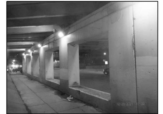
EXISTING LIGHTING: PIER 2 (Looking Southwest)
