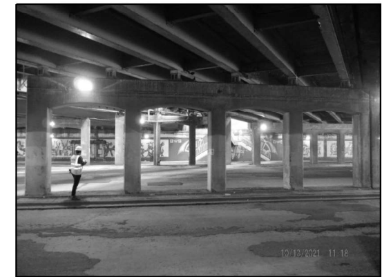
EXISTING LIGHTING: PIER 2 (Looking Southeast)
