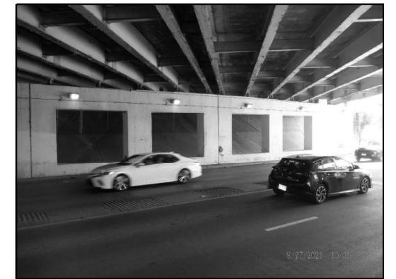
EXISTING LIGHTING: PIER 2 (Looking Southeast)
