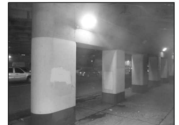
EXISTING LIGHTING: PIER 1 (Looking Southwest)
