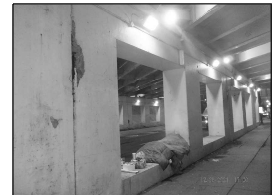
EXISTING LIGHTING: PIER 1 (Looking Southeast)
