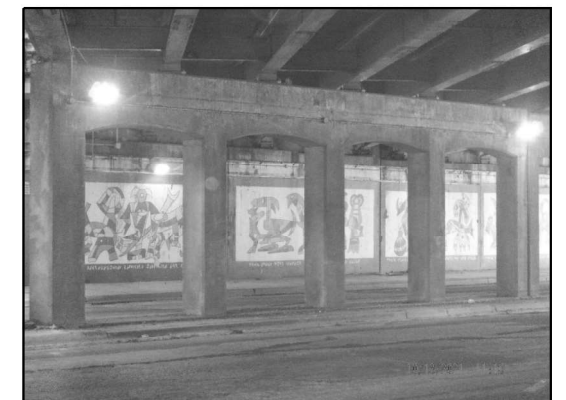
EXISTING LIGHTING: PIER 1 (Looking Southeast)
