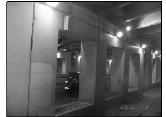
EXISTING LIGHTING: PIER 1 (Looking Southeast)
