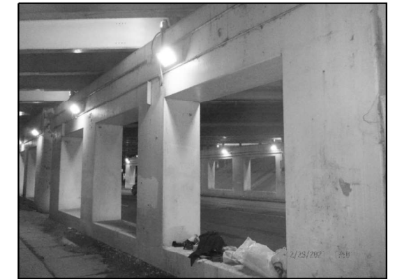
EXISTING LIGHTING: PIER 2 (Looking Southwest)
