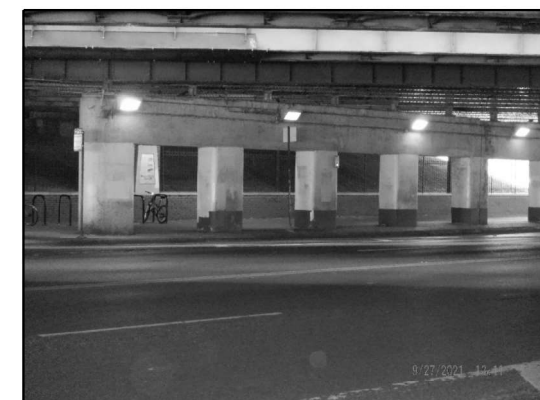
EXISTING LIGHTING: PIER 2 (Looking Southwest)
