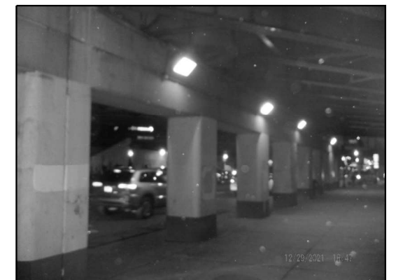
EXISTING LIGHTING: PIER 1 (Looking Southeast)
