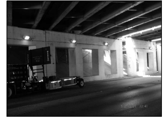
EXISTING LIGHTING: PIER 1 (Looking Southwest)
