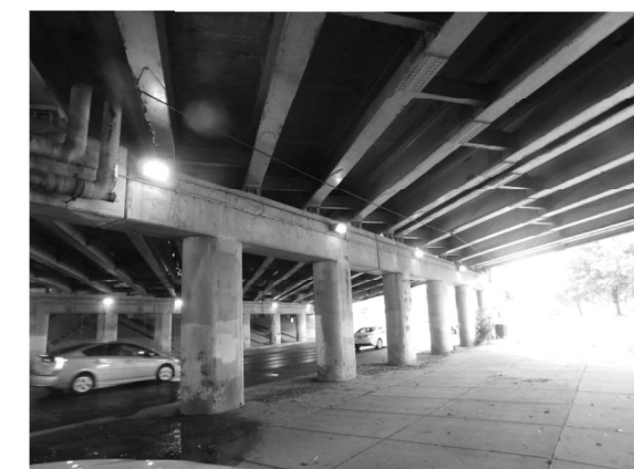
EXISTING LIGHTING: PIER 1 (Looking East)
