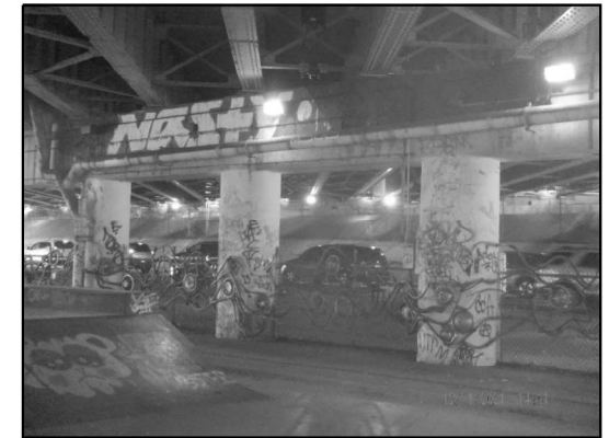
EXISTING LIGHTING: PIER 2 (Looking Southeast)
