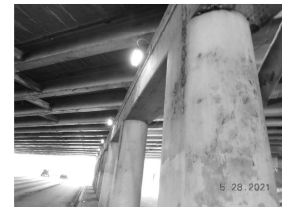
EXISTING LIGHTING: PIER 1 (Looking Southwest)
