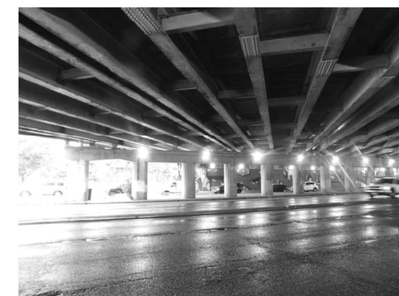
EXISTING LIGHTING: PIER 1 (Looking West)
