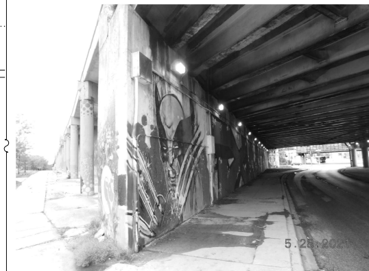
EXISTING LIGHTING: WEST ABUTMENT (Looking Northwest)
