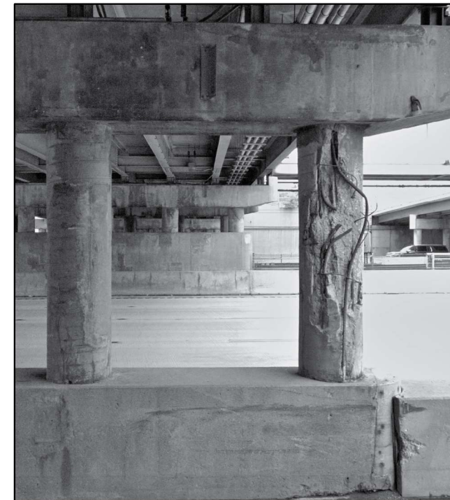
PICTURE OF PIER 4 DAMAGE
