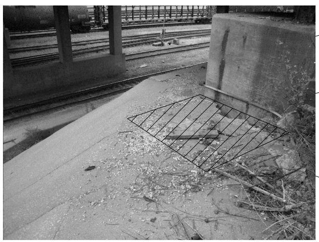
SLOPE WALL REPAIR AREA Looking South West
