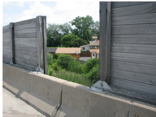
Photo 4. Missing Panel (NAW 3)
