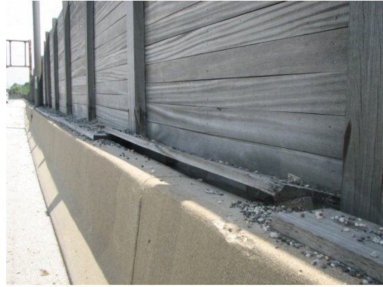
Photo 6. Loose Bot. Gap Board (NAW 3)
