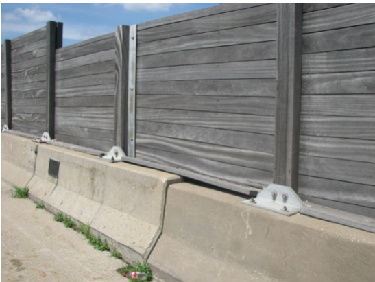
Photo 1. Loose Bottom Gap Board at SN 022-0138 (NAW 1)
