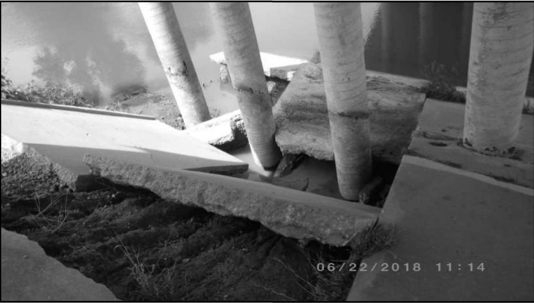
PIER 2 SLOPEWALL DAMAGE (Looking West)
