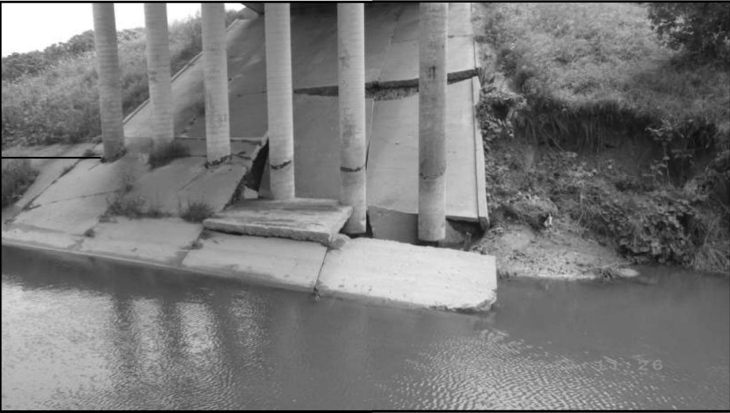
PIER 2 SLOPEWALL DAMAGE (Looking East)
